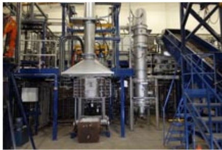
Advanced: Gasplasma's test facility in Swindon
